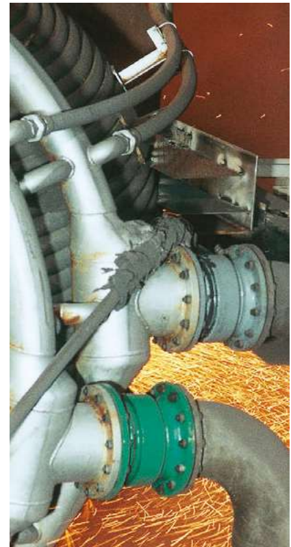
STENFLEX® Swivel Joint type DG-02L in cooling water line of exhaust pipe of furnace in a steel mill
